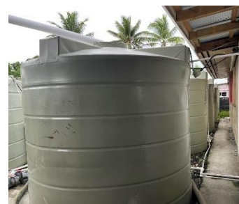
Circular rainwater tank in Funafuti. (Source: Tuvalu NAP Project-Mission (2024))
