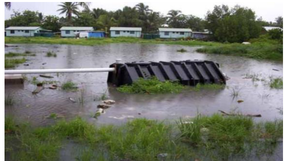
Septic waste system in Tuvalu's Vaifou settlement during a flooding event. (Source: Economics of liquid waste management in Funafuti, Tuvalu (2006))
