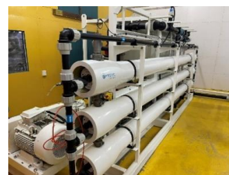
Desalination infrastructure in Funafuti. (Source: Tuvalu NAP Project-Mission (2024))
